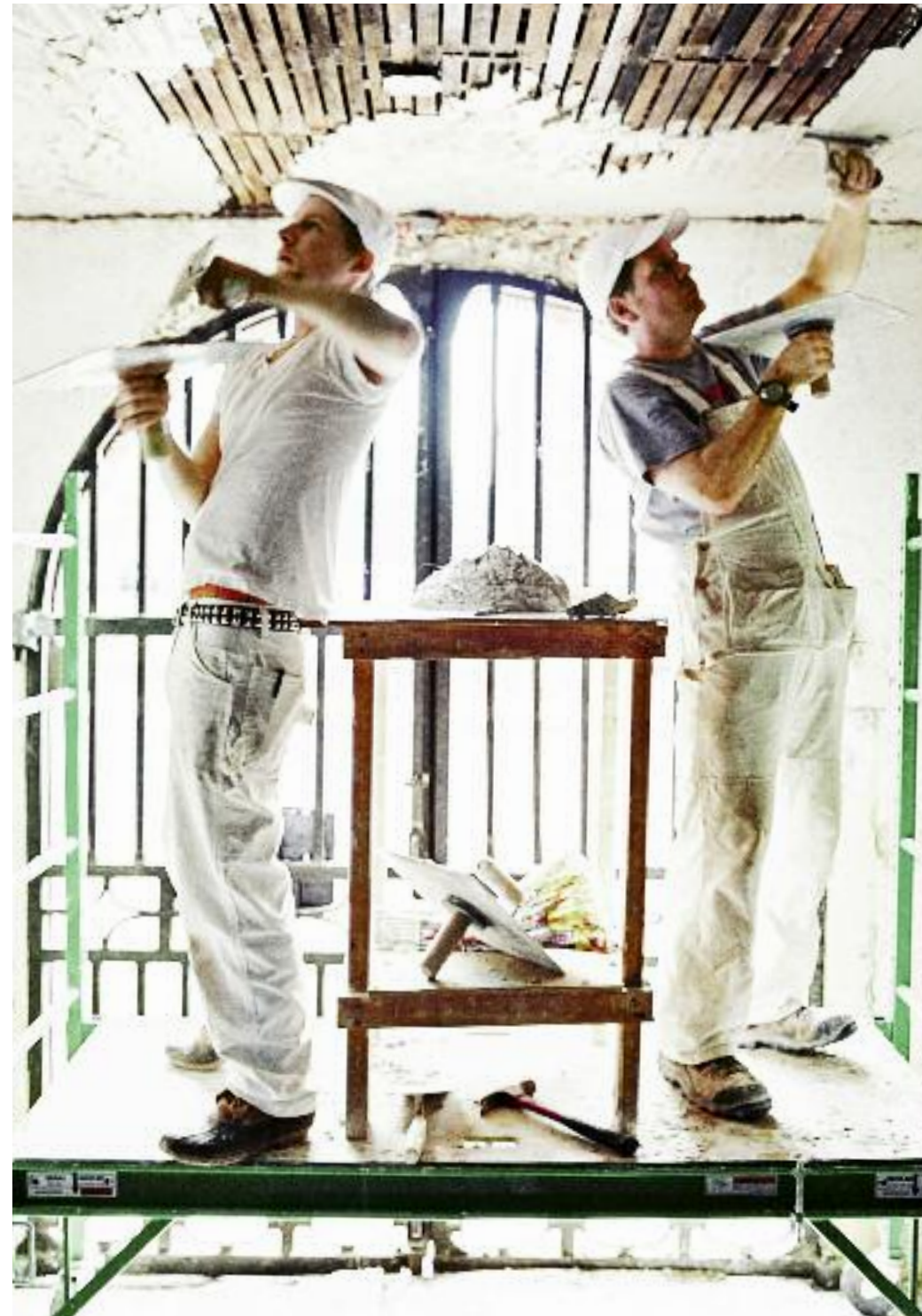
Students Mike Lauer (left) and Cody Donahue plaster the ceiling of the jail, which the college is slowly restoring with help from Save America's Treasures, a partnership between the National Trust and the National Park Service.
